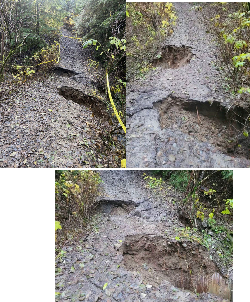
Major erosion around the culvert system has caused an unsafe and impassable section in the Cable Car – Fairground connection trail. This area requires a thoughtful and carefully considered approach to ensure the trailway does not slough or erode in the future.
